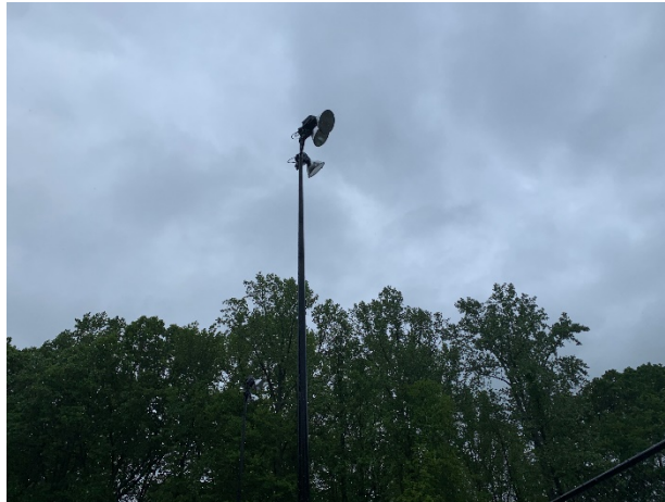
Light pole and fixture at the Tennis Courts
