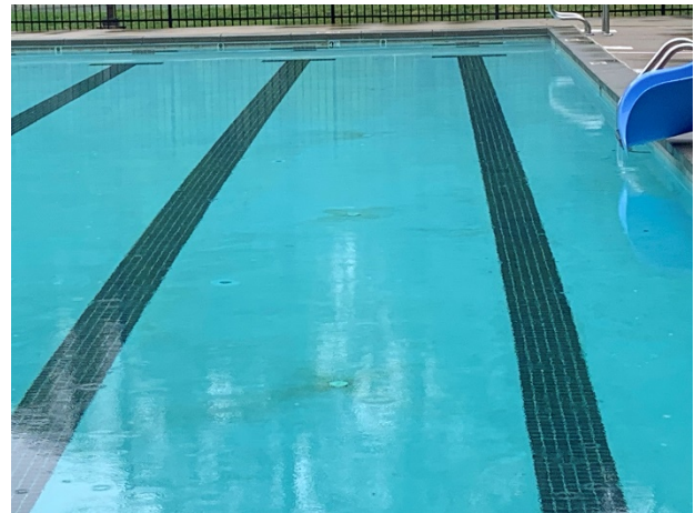
Stains around the drains evident
