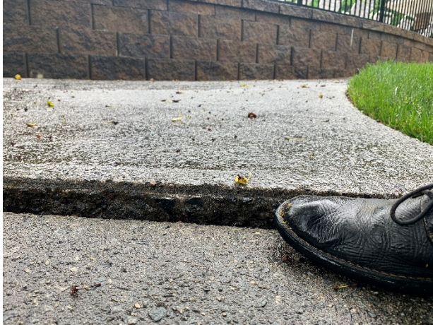
Trip hazards evident at the sidewalks – we recommend the Association fund these repairs through the operating budget
