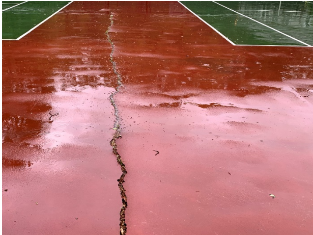
Severe cracks evident
